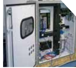
Control Systems with optional centralized SmartDolly and Automated Guided Vehicle routing capabilities, IT integration, and UL 508 panel build.
